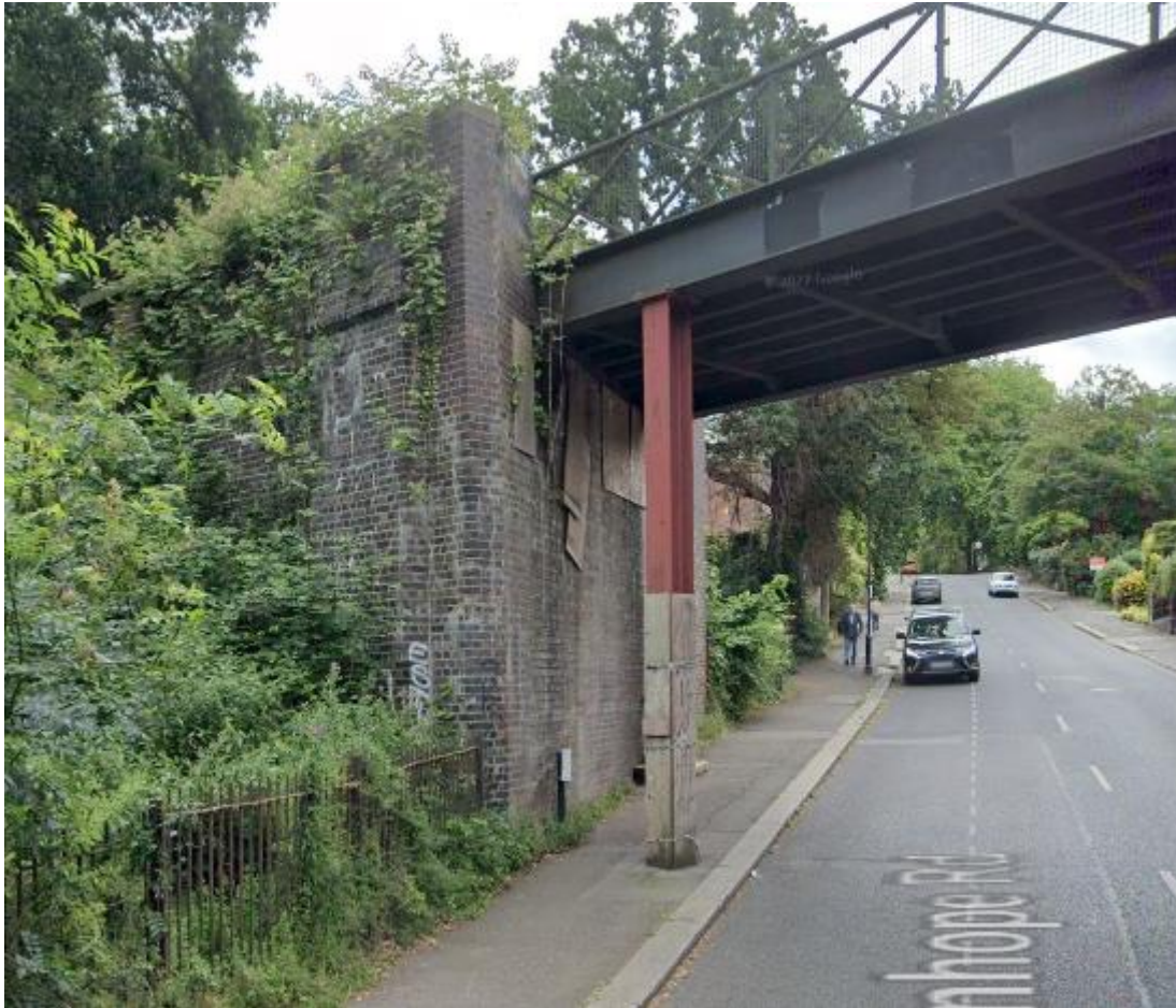
Figure 2: View looking south along Stanhope Road showing temporary structural props on east footway.
