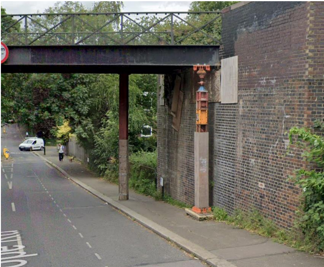
Figure 1: View looking north along Stanhope Road showing temporary structural props on east footway.
